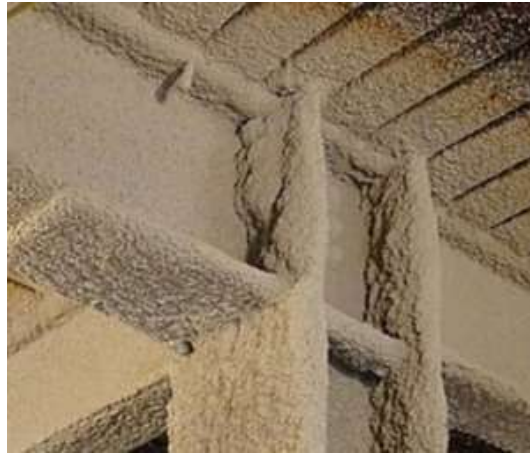
Figure 2. Spray-applied Fire-Resistive Materials (SFRM) 5
