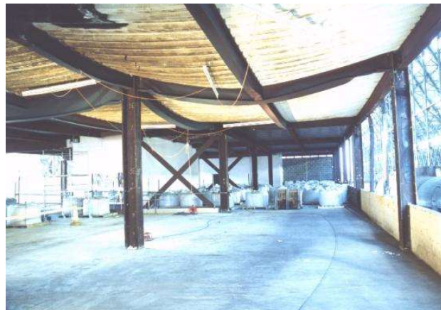
Figure 7. Beam Deflection after the Fire 10
